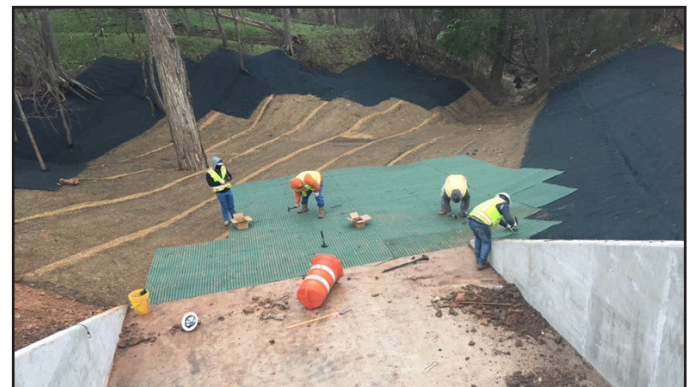
Before and after images of a wide channel managing storm discharge from the 6 ft culvert. The steep, meandering channel was stabilized with ShoreMax transition mat installed over permanent TRMs (bottom).
