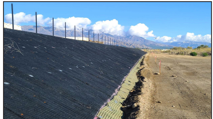
Progression of the installation of a permanent erosion control system on the Santa Clara River riverbank slope stabilization project.
