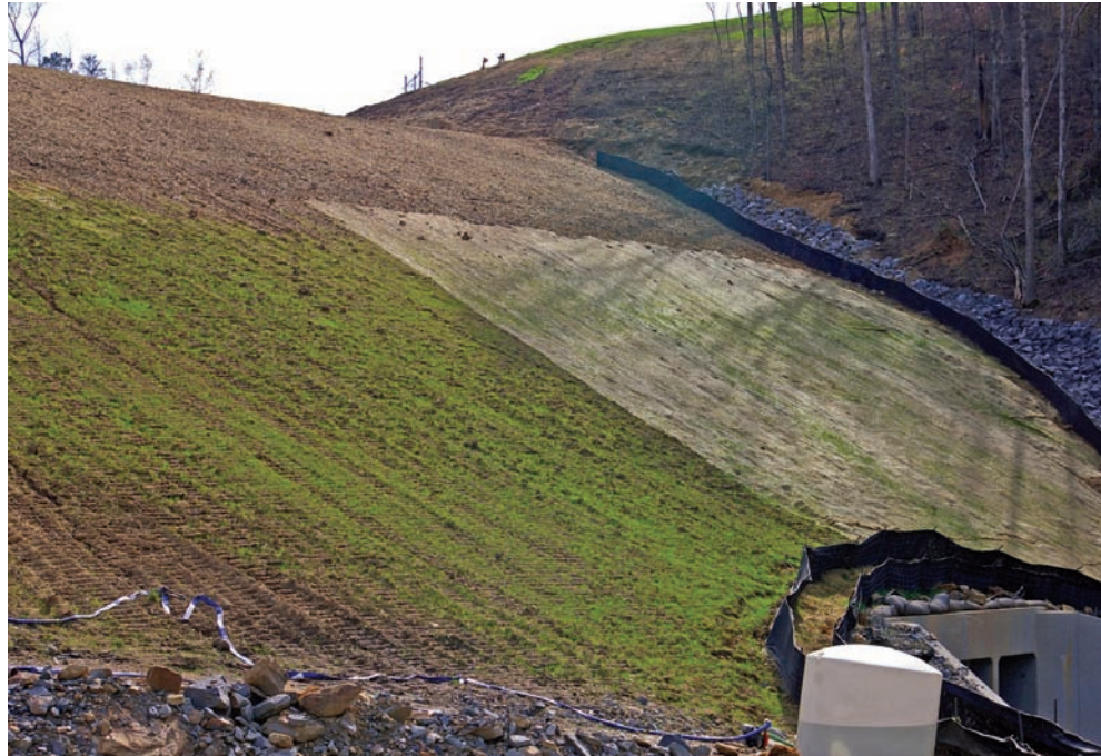
The ALDOT test site, which featured steep 2:1 roadside slopes with a 144-foot slope face, tested HydraCX2 (left) alongside several other erosion control products, including blown straw and a single-net straw erosion control blanket.
