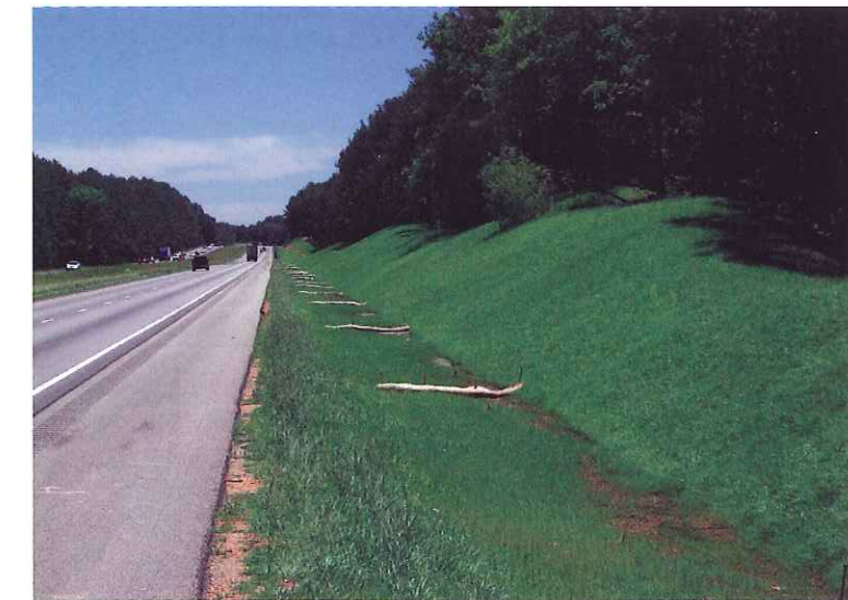
Full, lush grass growth was so noticeable that some motorists contacted the ALDOT to compliment them on restoring safety and beauty back to I-65.
