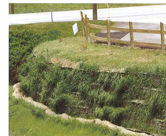
Photo 8 | The stabilized creekbank was designed to eventually blend into the surrounding landscape.
