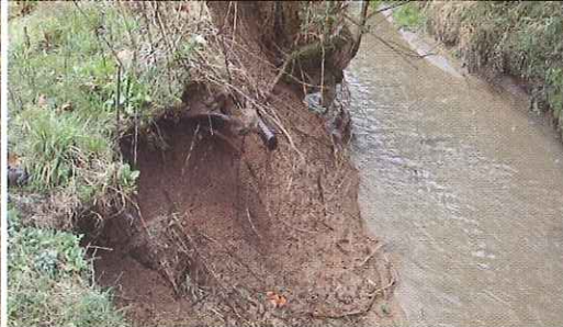
Photo 3 | Post-hurricane runoff accelerated creekbank erosion.
