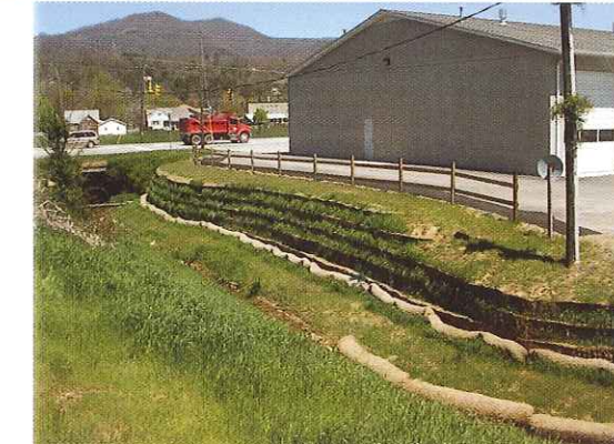
Photos 6 & 7 | A geosynthetically-reinforced MSE slope stabilized the creekbank adjacent to the Clyde Fire Station.
