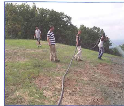
After 21 days of consistent rainfall, the crew forged ahead and began installation only 2 days later.
