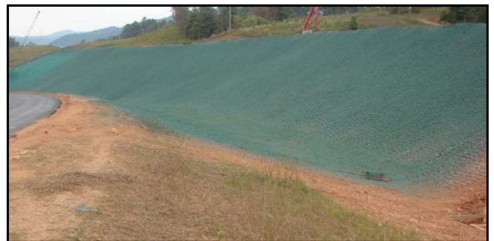
All the slopes were track walked prior to application of HydraCX 2 Extreme Slope Matrix (top), while the mulch was applied to the steep 1.5:1 slopes from two directions (bottom).
