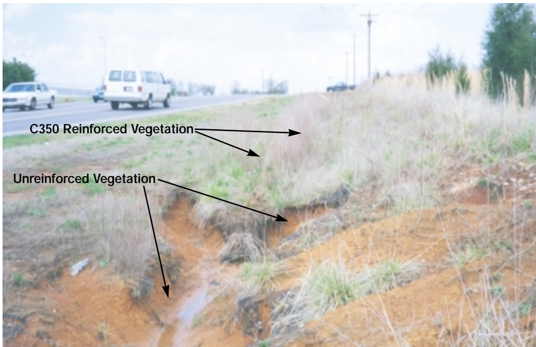
The C350 has afforded excellent erosion protection while assisting in the development and reinforcement of a dense stand of vegetation (upper portion of photo). However, re-seeding and mulching the section of the channel disturbed for crossroad construction was ineffective at stopping the erosion or allowing a good stand of vegetation to develop (lower portion of photo).
