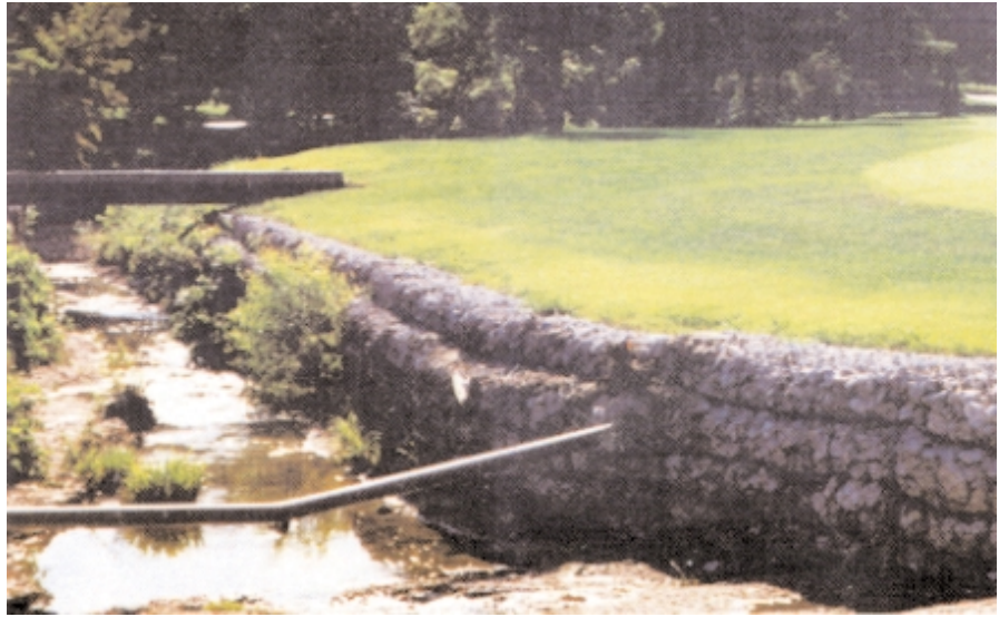
Wire gabion baskets encapsulate rock riprap to provide hard-armor protection and permanent stabilization for the banks of this perennial stream.
