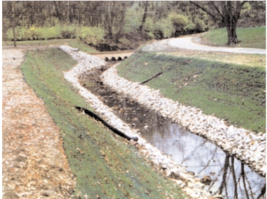
Swales and streambeds often require aggressive protection from erosion. Rock riprap and mat-reinforced vegetation provide stabilization for this channel.
